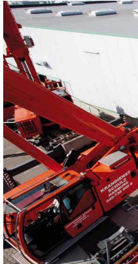
After two hours: the tank is already in place and the valve
