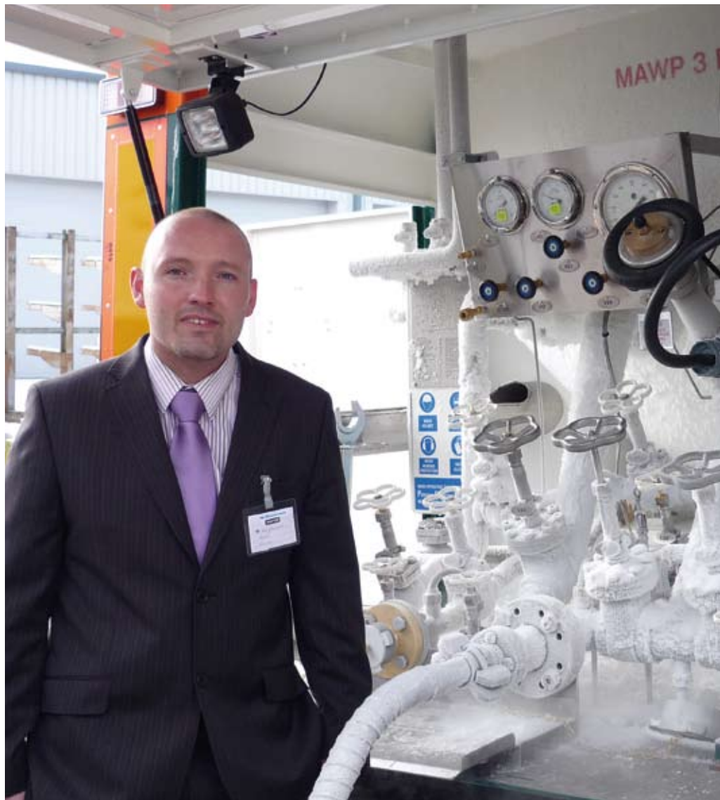
Barry Stewart and Jason Gill in front of a further trailer for Air Products, with series 09340 gate valves.
